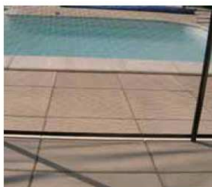
Fig. 7. The tension of the netting must be adequate, and the ground clearance according to the regulations
